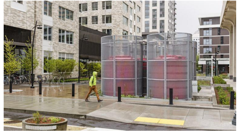
Hasslo on Eighth Development and onsite wastewater treatment and recycling plant in the Lloyd District, 2015
