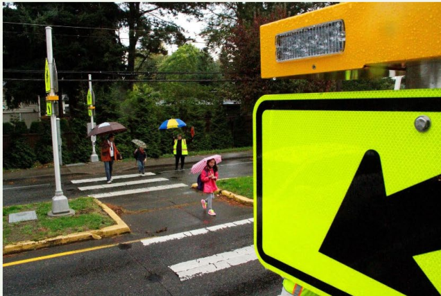
Rectangular Rapid Flashing Beacons (RRFB) on NE 116th St in Kirkland, WA.
