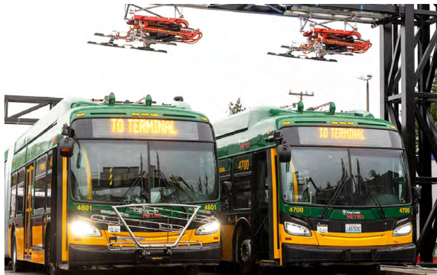
King County Metro electric charging
