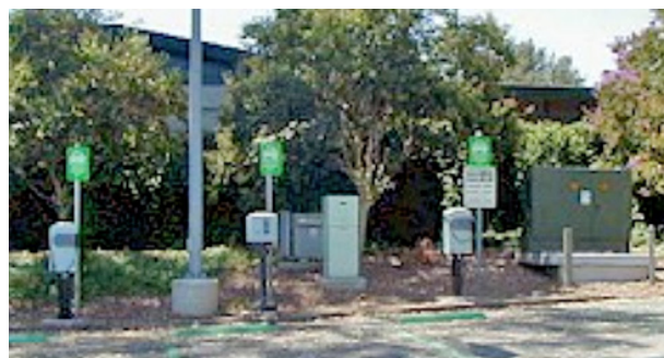
Figure 1. A typical pedestal-style charging station in a surface parking lot. Photo courtesy of ECOTALITY.
