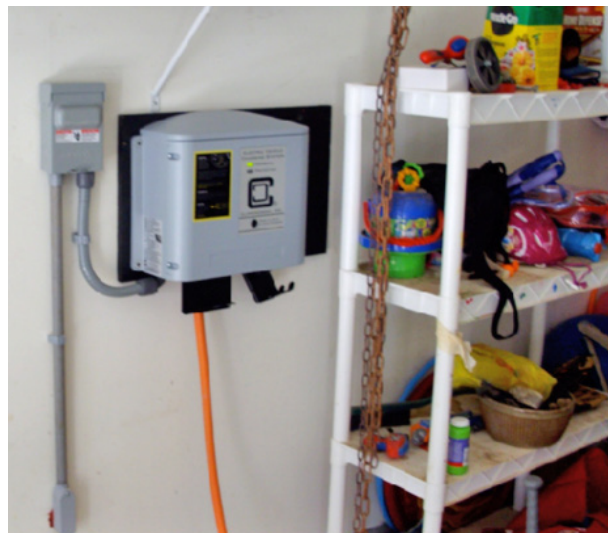
Figure 1. A typical wall-mounted Level 2 home charging station inside a garage. Photo courtesy of Clean Fuel Connection, Inc.
